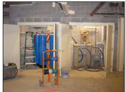
Water treatment system installed in a basement to mitigate the threat of contaminated water entering the city’s stormwater system
