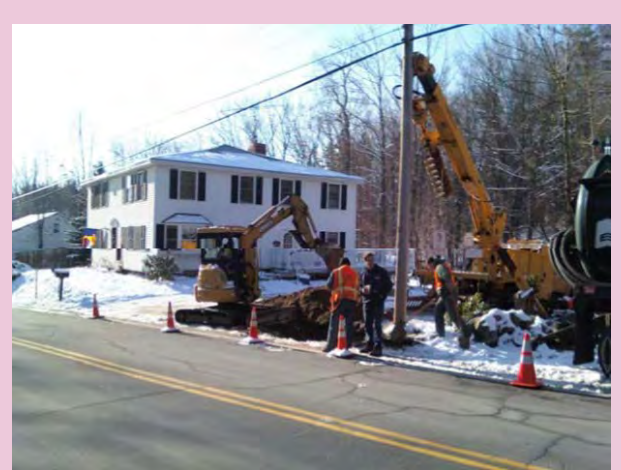
Excavation of abandoned gasoline tanks in a residential Lyndeborough neighborhood (Source: NHDES)
