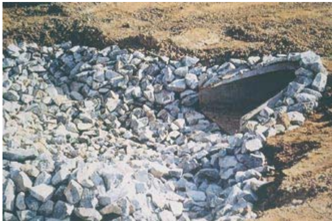
Excellent placement and construction of rock apron to dissipate flows from culvert outlet. Area needs seeding and mulching.
