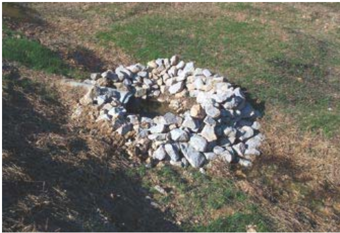
Very good application of mixed rock for culvert inlet ponding dam. Mixing rock promotes better ponding, drainage, and settling of sediment.
