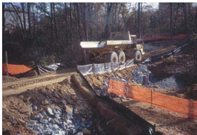
Good use of silt fence, straw, rock and other practices for temporary stream crossing. Any work in stream channels—such as installation of culverts
