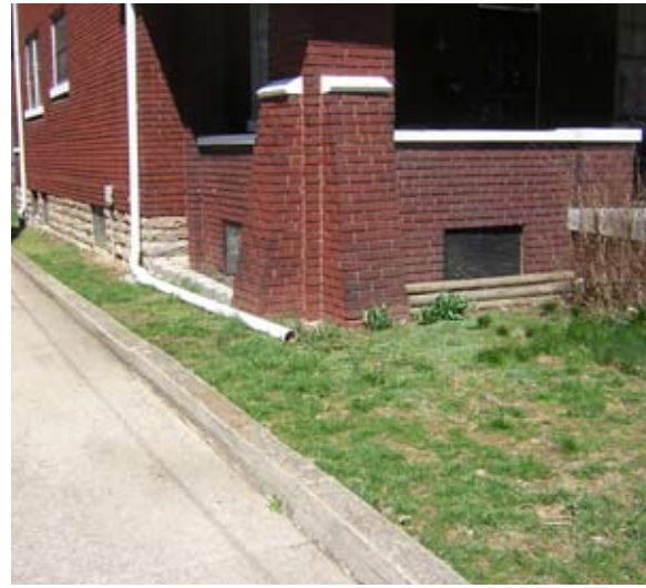
Figure 4-59: A residential example of downspout disconnection in Covington.
