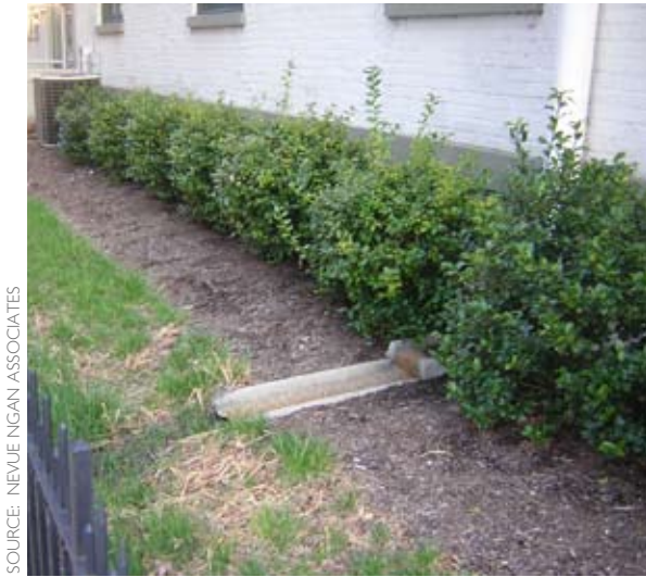
Figure 4-58: An office building in Covington has disconnected roof downspouts that allow water to flow into a landscaped area.
