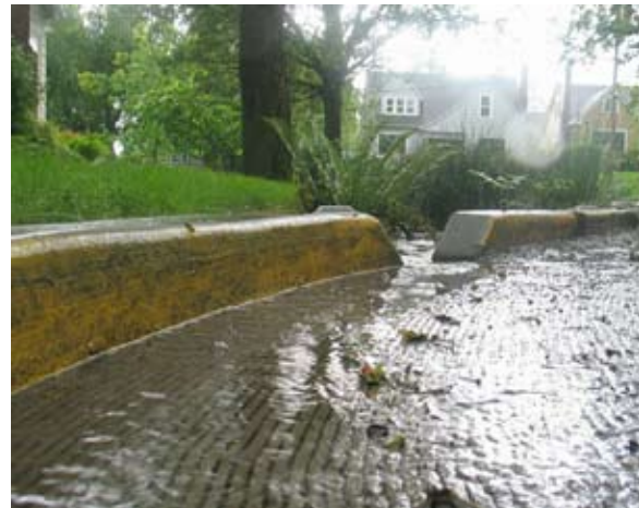
Figure G-2: A typical curb cut used to allow water to enter a stormwater curb extension.
