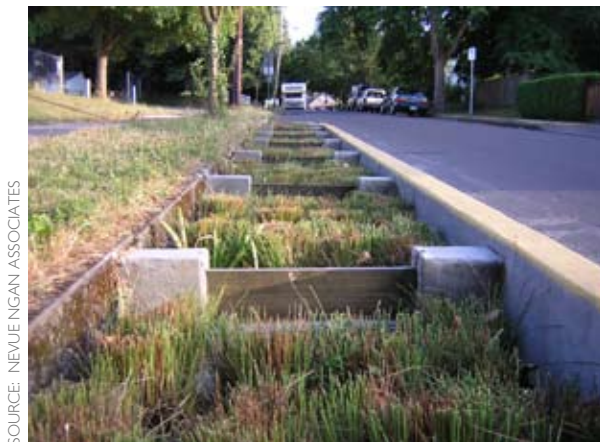
Figure E-3: Closely spaced check dams help terrace the interior landscape of this stormwater curb extension project. The slope of this street is approximately 6%.
