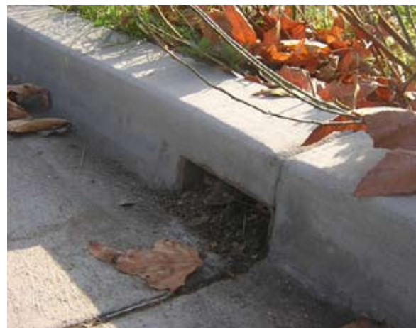
Figure G-3: This notched curb cut is way too small and constantly overloaded with sediment.
