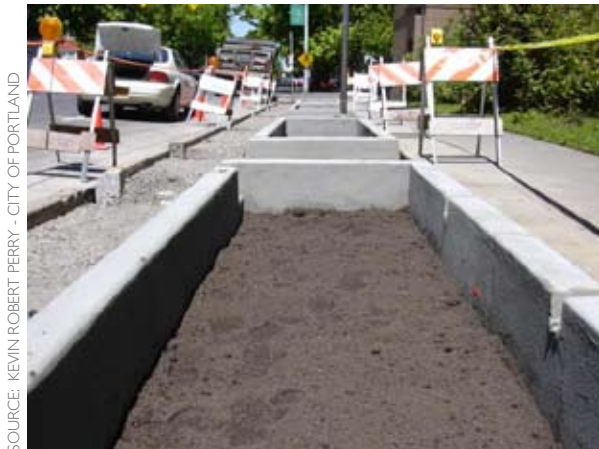
Figure L-2: New imported topsoil is placed within a planter. Soil is graded 2" lower than finish grade to account for a mulch layer.
