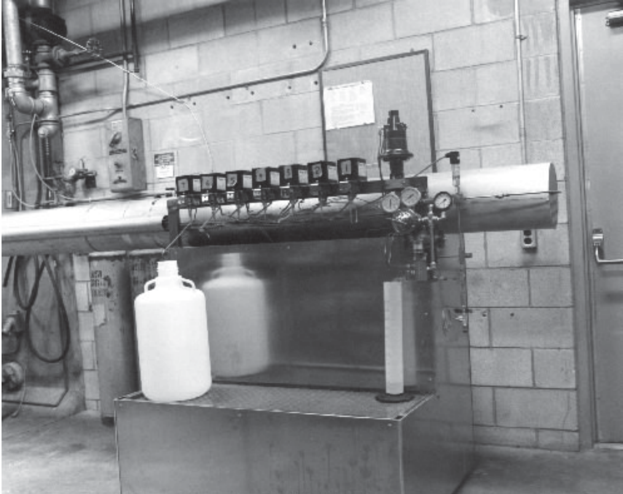
Figure 18. Photograph of pressure control subsystem
