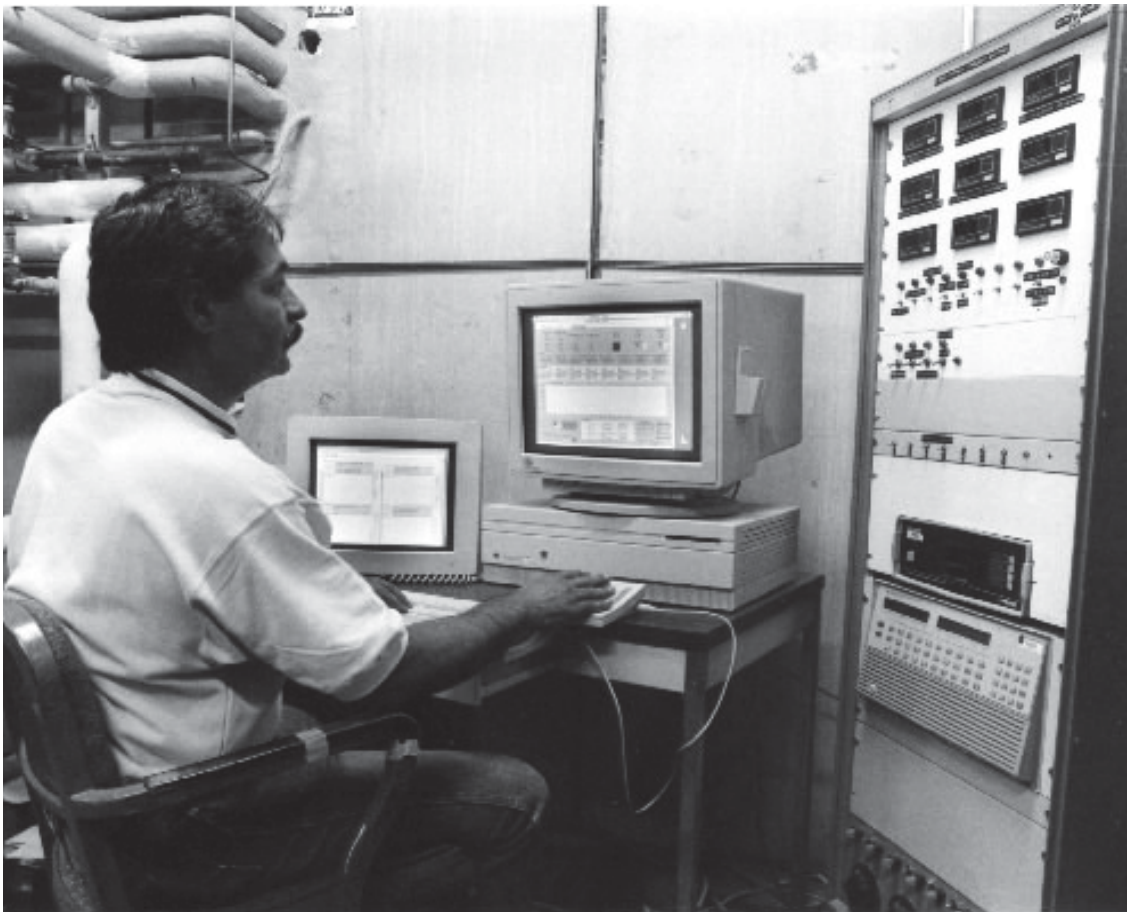
Figure 19. Photograph of data acquisition and control subsystem
