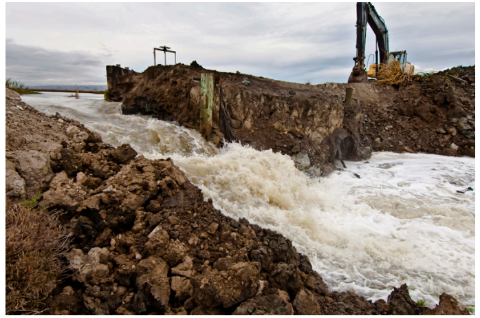
South Bay Salt Ponds, Pond A17 levee breach-opening to tidal flow to restore tidal wetlands (October 31, 2012). Photo: Judy Irving.
