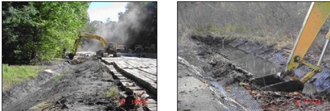
Figure 2-7 Creating a diversion channel around Area G using a tracked excavator (left). Construction of diversion channel around Area F (right).
