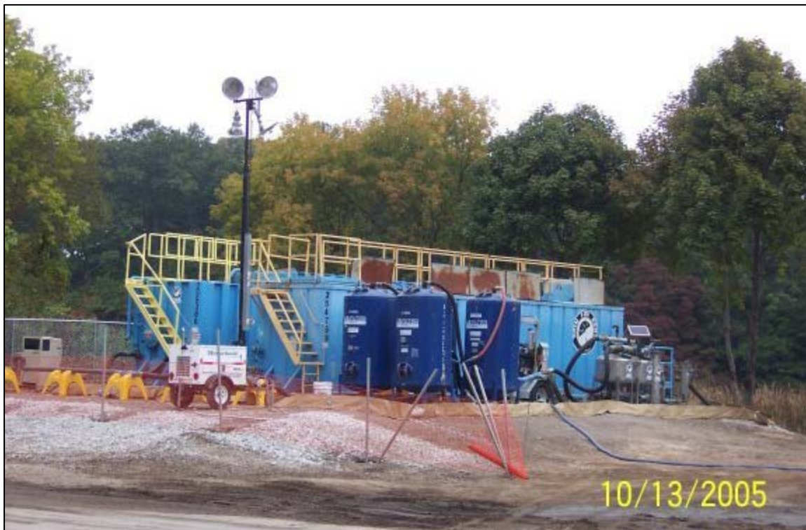
Figure 4-2 On-site treatment system
