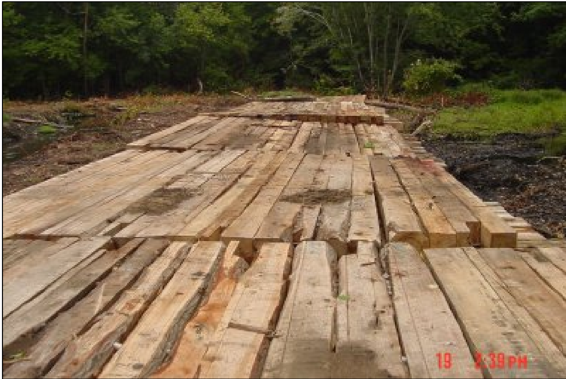
Figure 2-4 Timber swamp mat access road to Ruddiman Creek Main Branch remediation area
