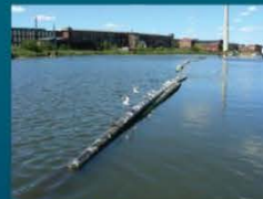
Floating and submerged pipelines
