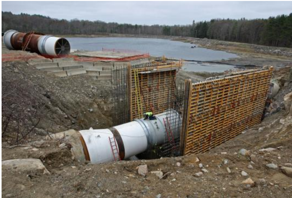
Repairs underway at damaged Hultman aqueduct in Weston, Massachusetts. The pipe in the background is from the damaged aqueduct. (Source: Jim Davis, Boston Globe)
