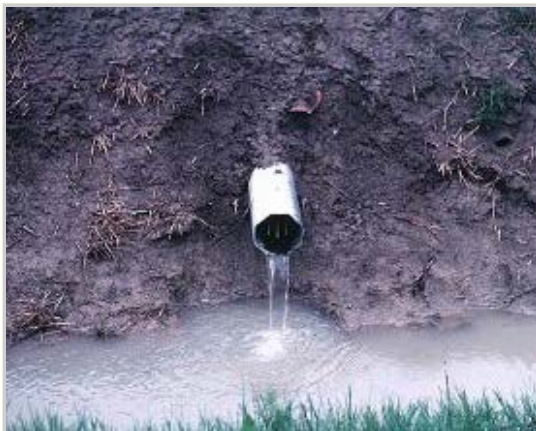
Drain tile outlet to a drainage ditch Source: Purdue University
