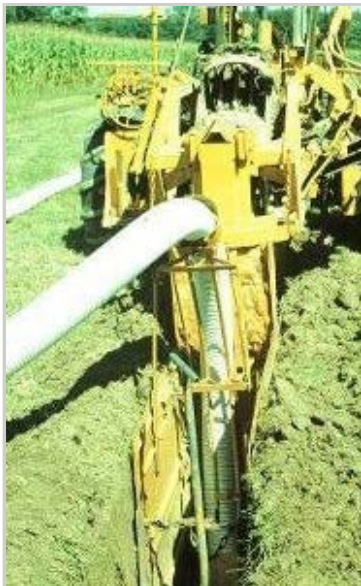
Trenching machine used by drainage contractors to install subsurface drainage tile (shown in white) Source: Purdue University
