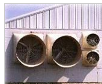
Mechanical ventilation in grow-finish building Source: Purdue University
