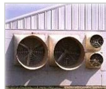
Mechanically ventilated building Source: Purdue University
