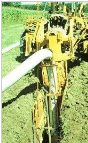
Trenching machine used by drainage contractors to install subsurface drainage tile (shown in white) Source: Purdue University
