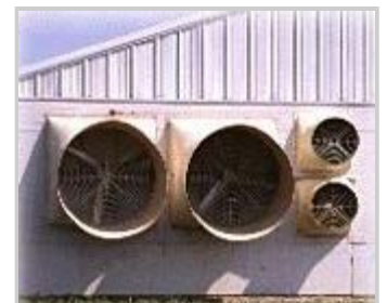
Mechanically ventilated building Source: Purdue University
