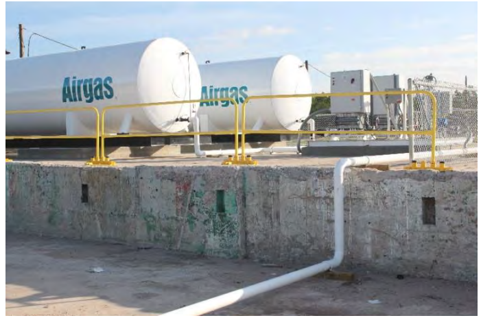
Right: 50-ton CO 2 storage tanks
