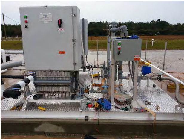
Left: 105-kW process vaporizers.
