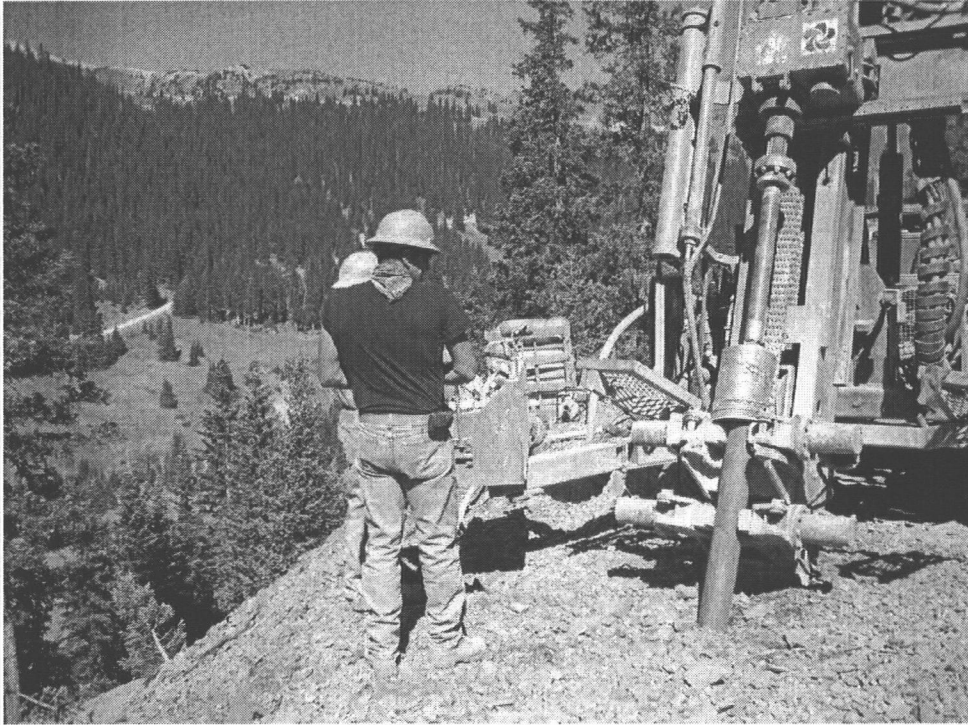
Photo 21 Drill rig on site drilling well RBMW01. Note ODEX surface casing being advanced.
