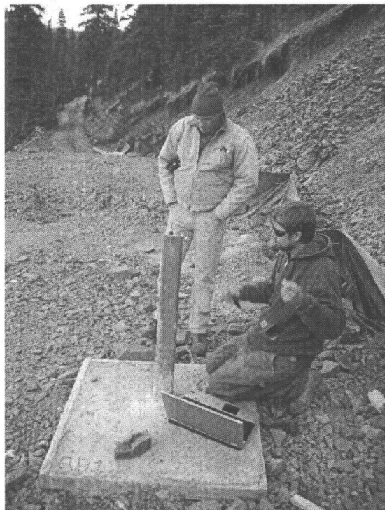
Photo 42 Initial programming of pressure transducer at RBMW01. Note drill pad and well apron. Silt fence emplaced along the upslope side of the drill pad.
