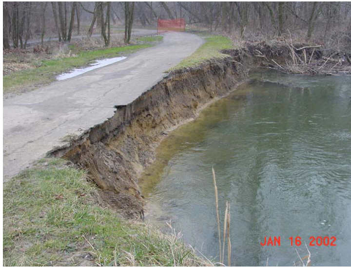
Figure 3.14 Bank Erosion in Sterling Heights Park. Source: MDNR
