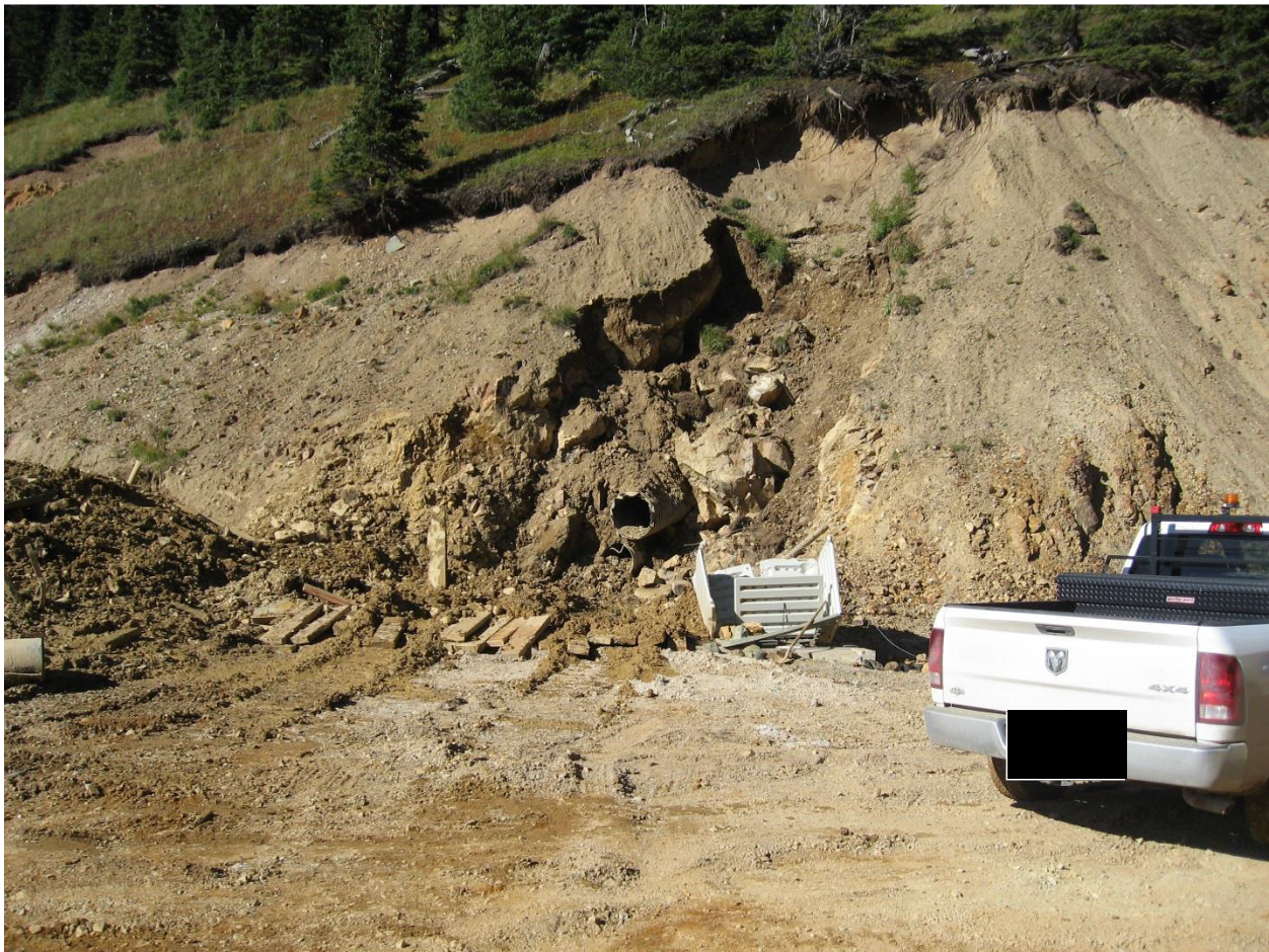
Gold King Mine – 9/11/14: collapsed adit pipe near roof of the adit/tunnel.
