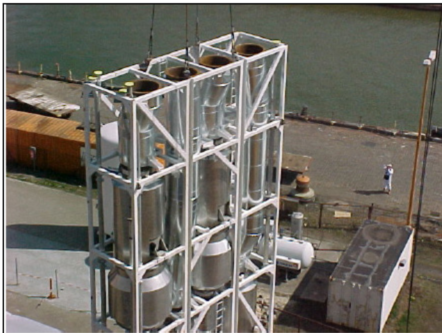
Figure 2-6. The EcoSilencer® Scrubber Installed on the Pride of Kent 5
