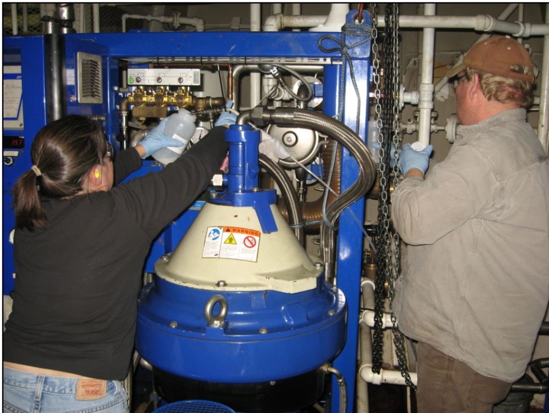
Figure 2-2. Sampling of Bilgewater from a Bilgewater Treatment System
