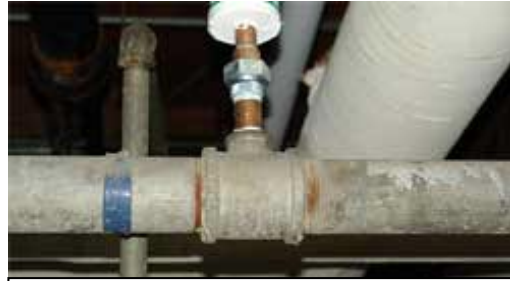
Typical iron/brass connection linked to elevated arsenic levels at some Seattle Public School drinking water fountains.
