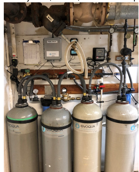
Figure 10. DI use in Buildings 20 and 47/49 is monitored using flow totalizing meters.
