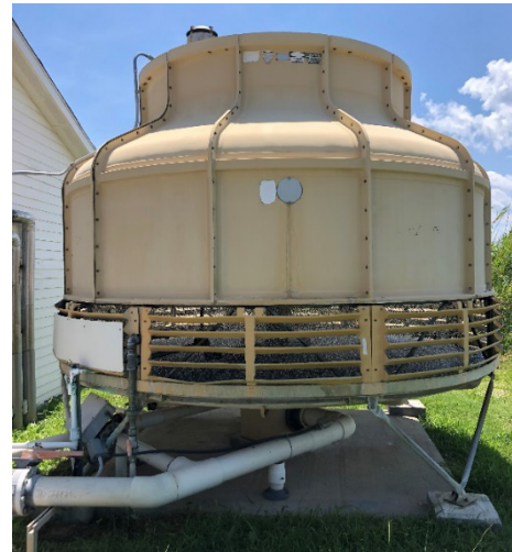
Figure 7: A 250 ton cooling tower serves Building 20.
