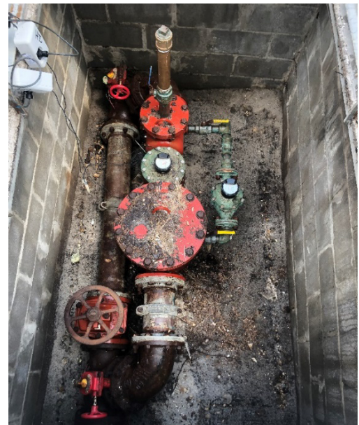
Figure 2: The GEMMD has high flow and low flow meters that totalize all potable water supplied by the ECUA. The meter is located below grade prior to going over the causeway to the GEMMD.
