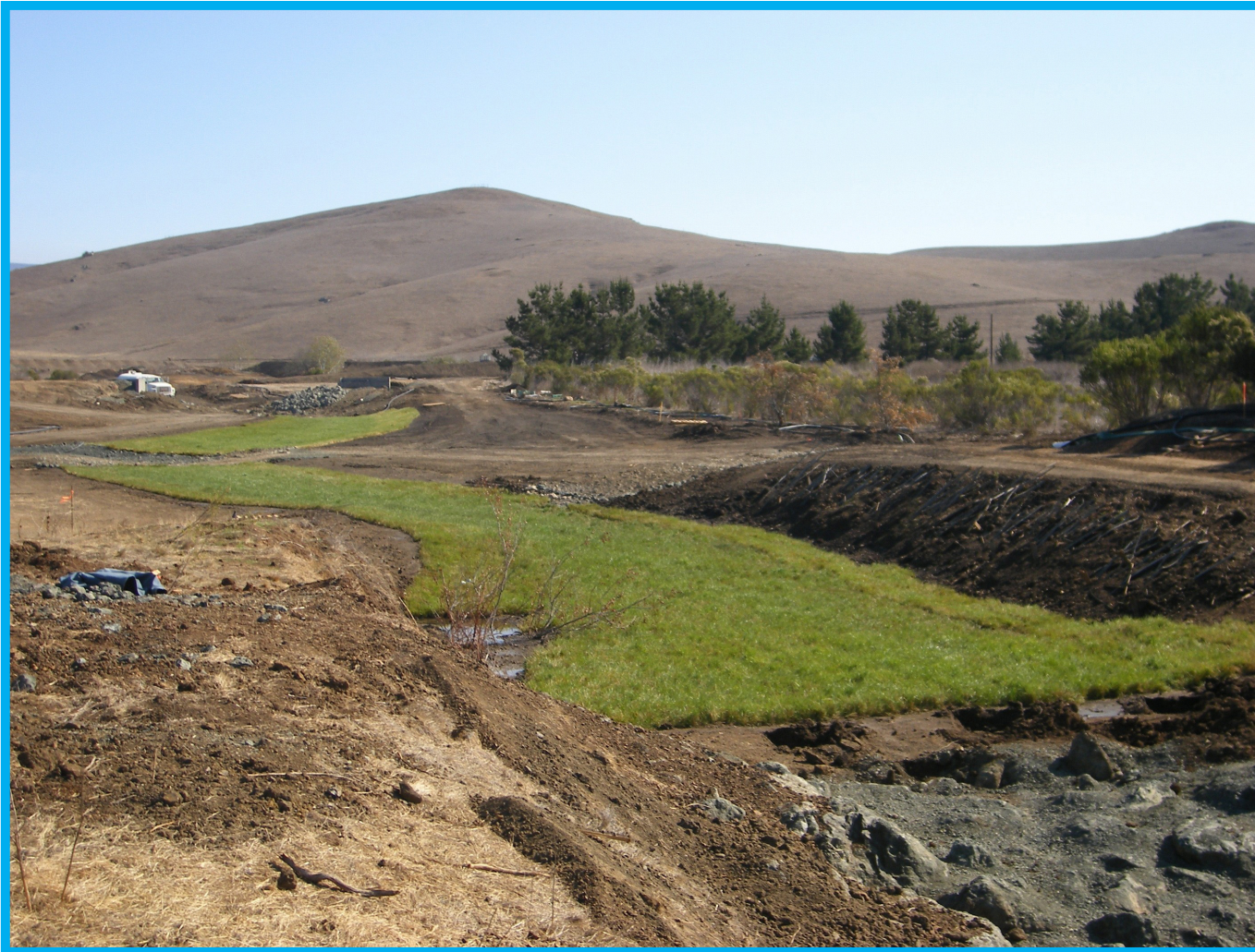
A view of the living channel liner installed. Photo: Jon Hall, MBNEP
