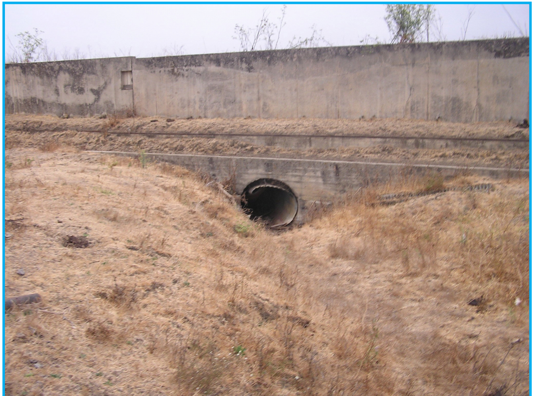
A dysfunctional culvert and retaining wall carry a tributary to Walters Creek. Photo: Jon Hall, MBNEP
