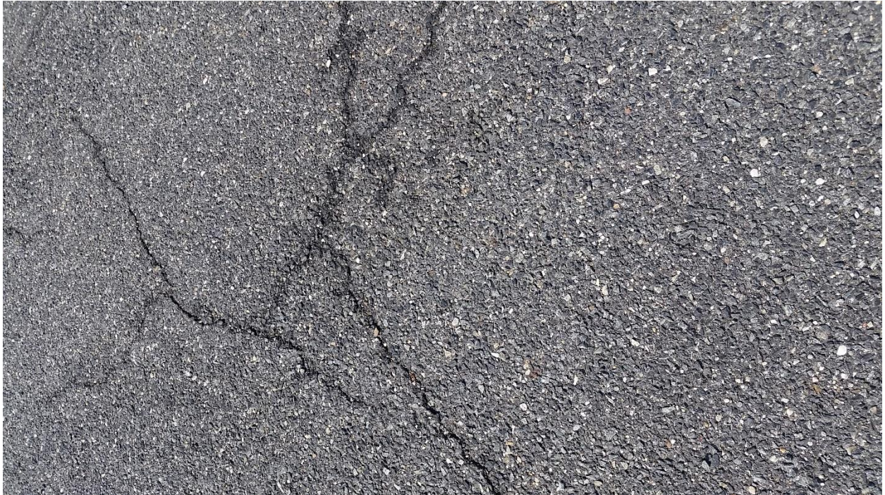
Picture 7: Cracks near North Corner of Cap
