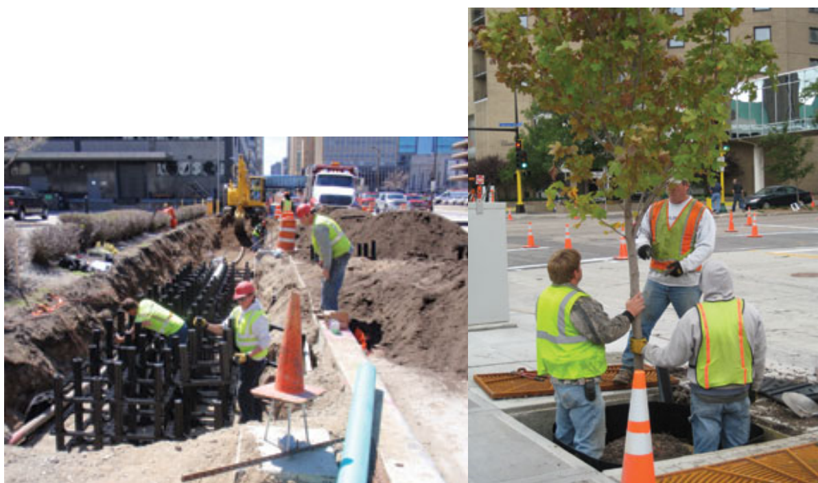
Figure 3-16. Under-sidewalk bioretention provides robust street trees as stormwater management benefit in the Minneapolis MARQ2 project.
