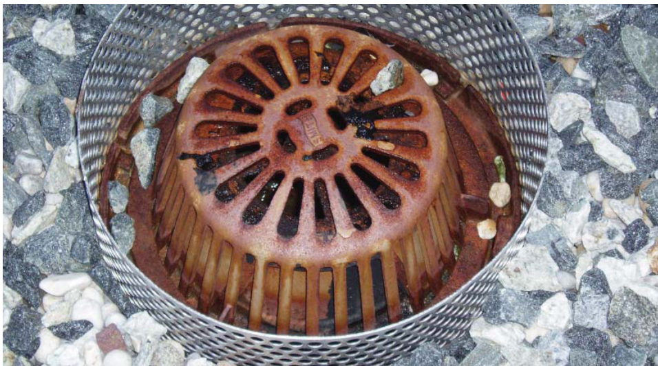
Blue roof drain installed by the SCA on PS 12 (Photo credit: Council on the Environment New York)
