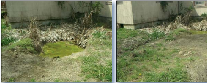
Figure 2. Watershed partners worked with a residential landowner to repair a failing septic system (left: before, right: after).
