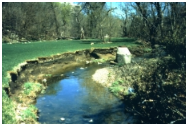
Streambank erosion, 1994 (Waukegan River, Illinois).
