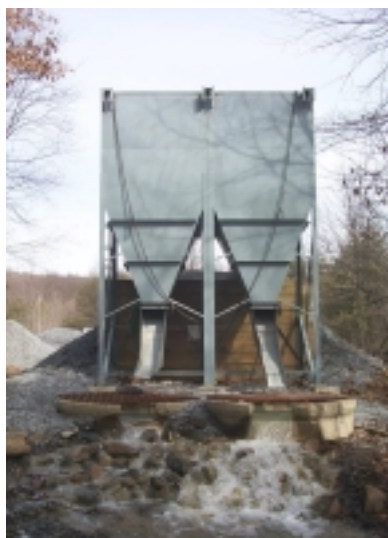
Limestone diversion wells to neutralize acidic coal mine drainage (Swatara Creek, Pennsylvania).
