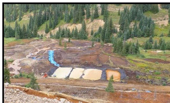
Temporary treatment ponds near Gold King Mine
