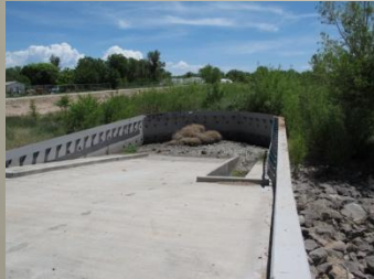
Sanchez Farm Inlet (trash/sediment removal structure)
