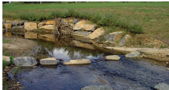
Figure 2. Post-restoration: Rock toe and vane, cross vane, and rootwad installed for bank stabilization, hydrologic direction, and grade control. (Source: DNREC 2005)
