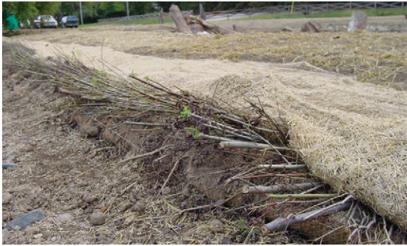
Figure 3. Post-restoration: Live riparian willow sprigs ( Salix sp.) and coir matting installed for bank stabilization and to establish a riparian buffer. (Source: DNREC 2005)
