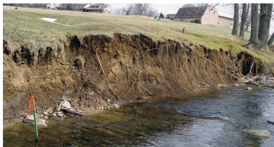
Figure 1. Pre-restoration: Severe bank erosion along the Pike Creek mainstem at the Three Little Bakers Golf Course. (Source: DNREC 2002)
