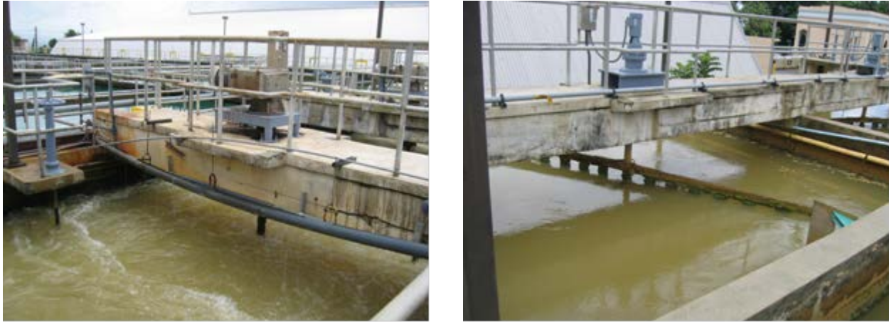
Figure 3-2. Guaynabo WTP Flocculation Basins During Mixing (Left) and Settling (Right)
