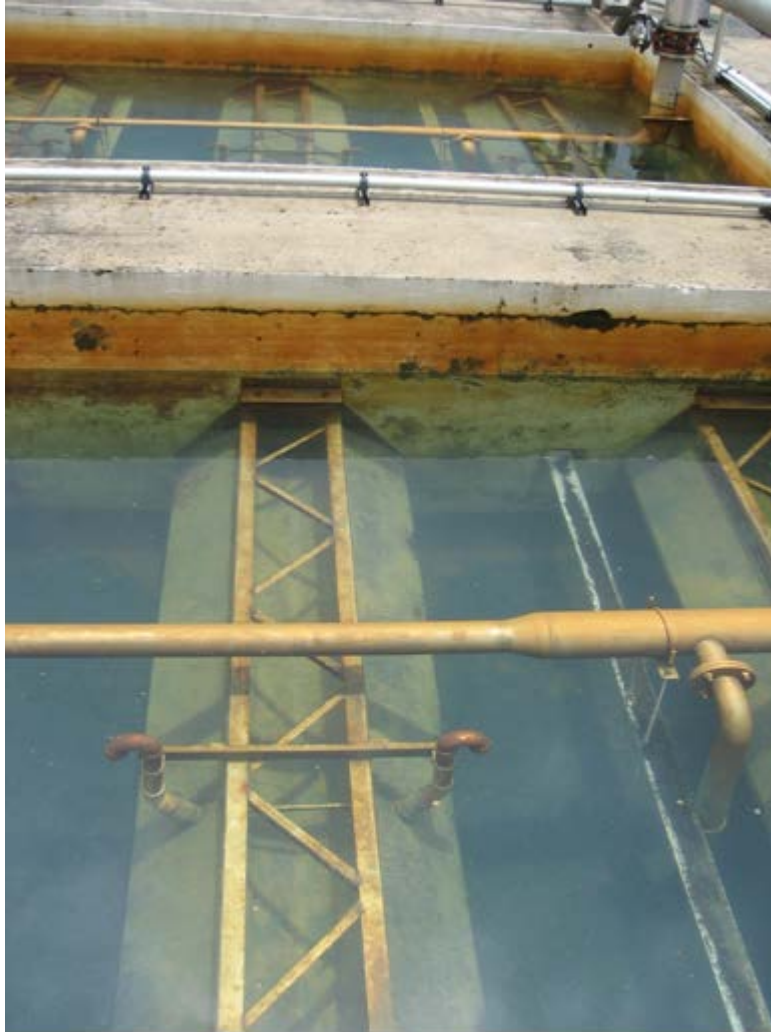
Figure 3-4. Guaynabo WTP Filters
