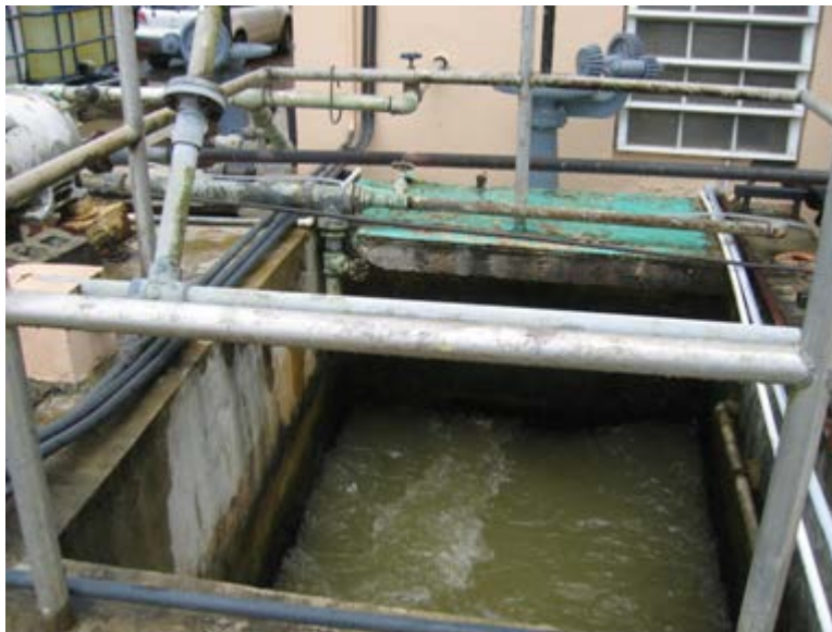
Figure 3-1. Guaynabo WTP Intake and Rapid Mix Tank
