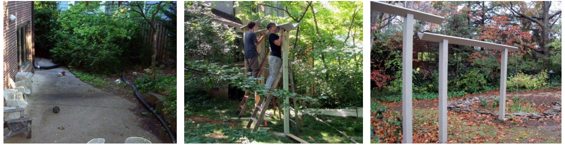
Figure 1. Jeff and Joan Harn's home has a walk-out patio (left photo). The poorly drained property was under constant threat of basement flooding before the project. Because the only available space for a rain garden was located uphill from the patio and existing downspouts, the homeowners opted to build a short aqueduct to deliver roof runoff to the rain garden (middle and right photos).
