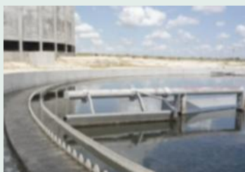
Secondary sedimentation basin at the new 5.7 MGD Reynosa wastewater treatment plant.
