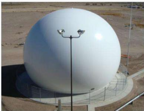
A methane capture system in Mexico at Ciudad Juarez's South Wastewater Treatment Plant harvests methane from the anaerobic digestion treatment process.
