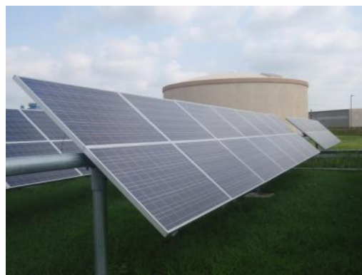
New solar panels in Mexico at San Benito's drinking water treatment plant reduce energy costs, which are a major expense for most water utilities.
