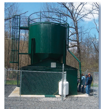
Figure 2. This lime doser was installed as part of the Three Fork Creek restoration.
