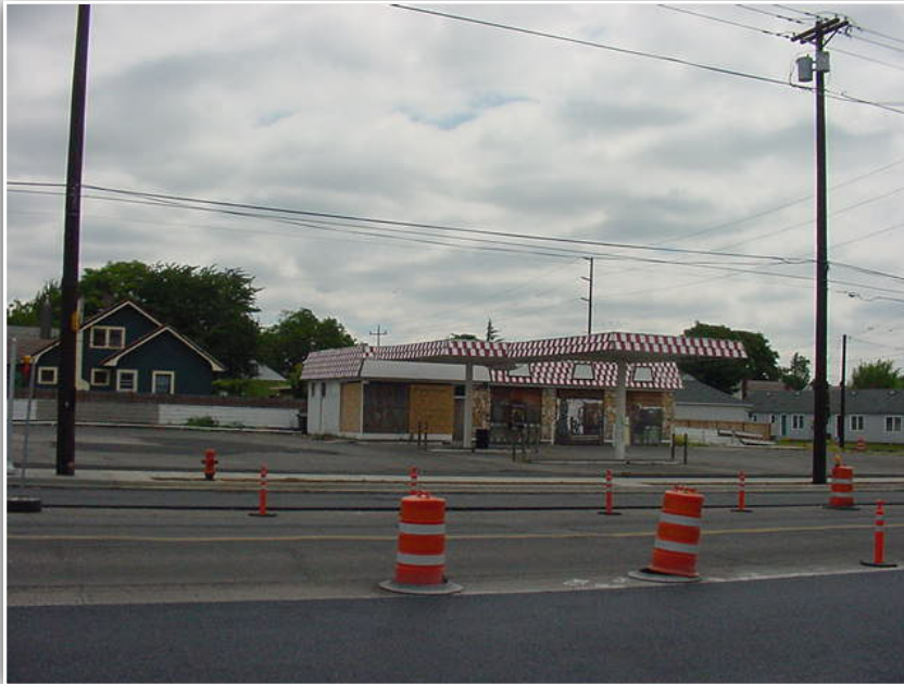
This Abandoned Gas Station was the focus of the Design Charrette at the Brownfields 2003 national conference
