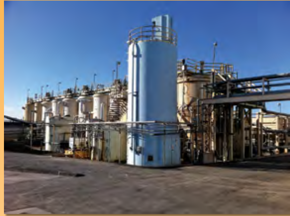
Tronox wastewater treatment system.
