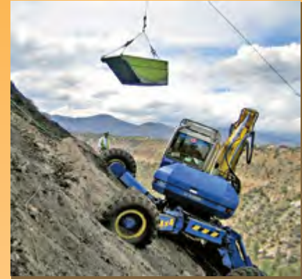
Equipment operates on steep canyon. Photo courtesy of Los Alamos National Laboratory.
