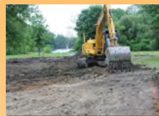
Heavy equipment removes lead tainted dirt from nearby park. Photo courtesy of Reading Eagle.
