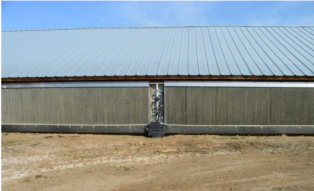
Figure 6. Evaporative cooling pads in the sidewall near the E end of one of the barns.
