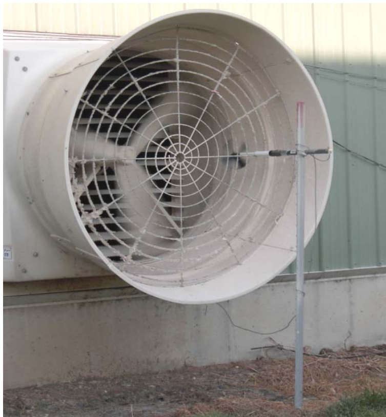
Figure 1. Model 27106RS Impeller Anemometer installed on a post on the exhaust side of a ventilation fan (Hoff et. al. 2004)
