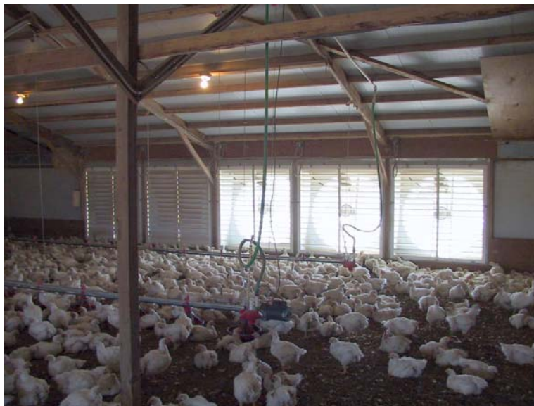
Figure 3. The bank of 48-in fans in the N sidewall of barn 10.
