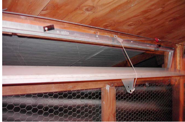
Figure 3-2. Example House Air Inlet
