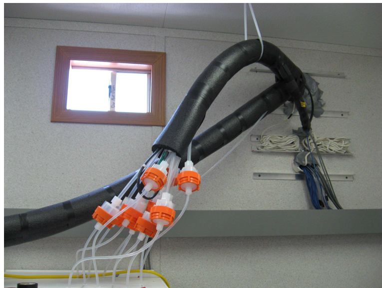
Figure 4. Bundled and insulated tubing and uninsulated cables and wires entering the raceway from the OFIS (Photo courtesy L Cai, Iowa State University).
