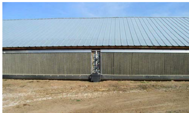
Figure 3-4. Evaporative Cooling Pads
