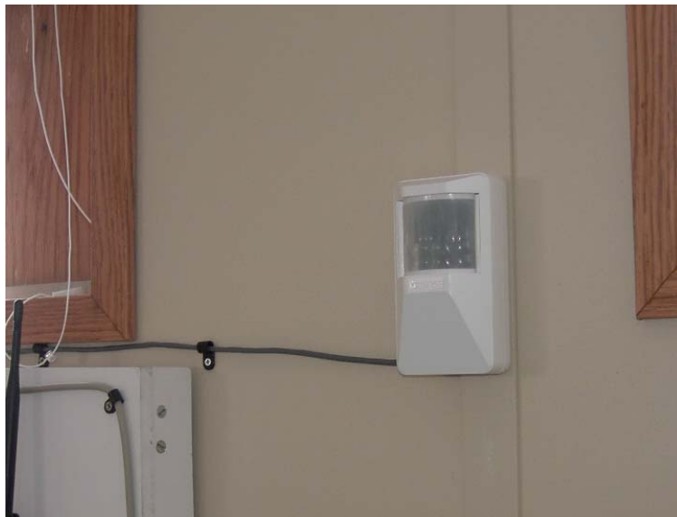
Figure 4. Activity sensor installed at the end wall inside an instrument shelter.
