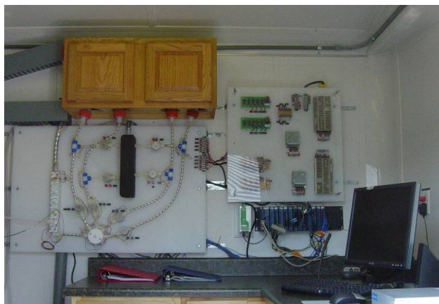
Figure 6.6. View of hardware required to run pollutant sampling system.
