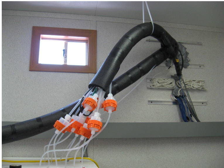
Figure 4. Bundled and insulated tubing and uninsulated cables and wires entering the raceway from the OFIS (Photo courtesy L Cai, Iowa State University).
