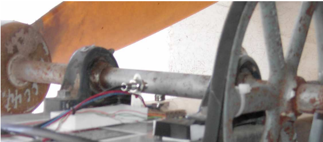
Figure 1. RPM sensor mounted perpendicular to fan shaft.
