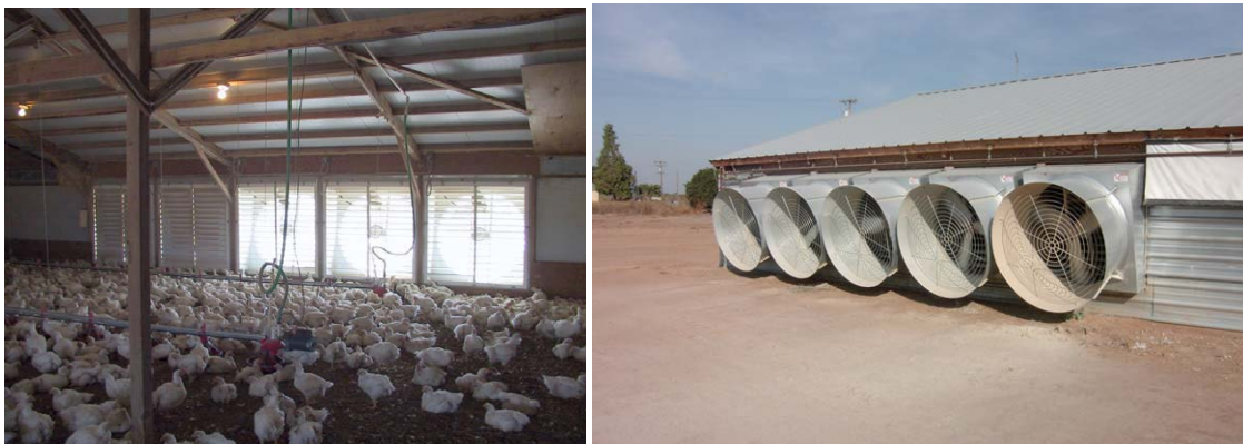
Figure 3-3. Bank of 122-cm (48-inch) Fans (left, view from inside of house) and (right, view from outside of house)
