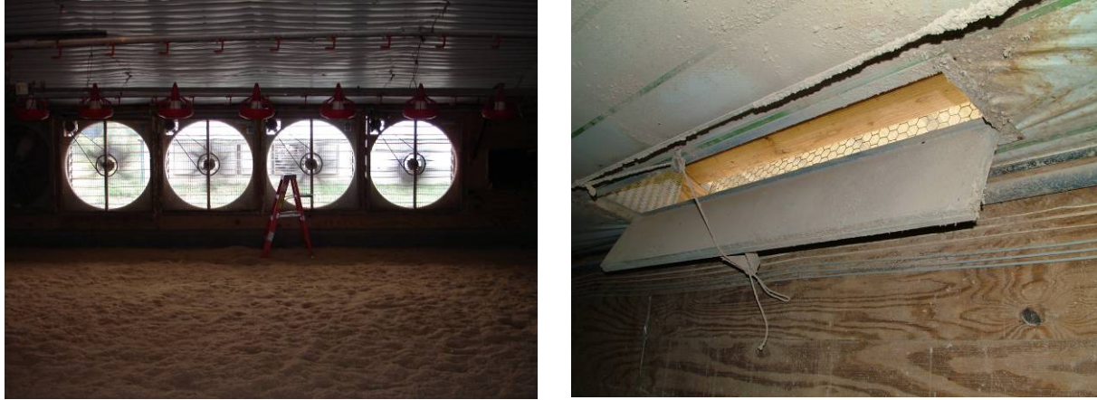
Figure 3-7. Tunnel Fans and Box Air Inlets
