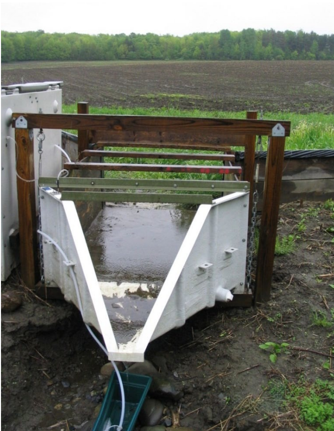
Figure 3-6. 2-foot (0.6 m) H-flume in place for edge-of-field monitoring, East Montpelier, VT
