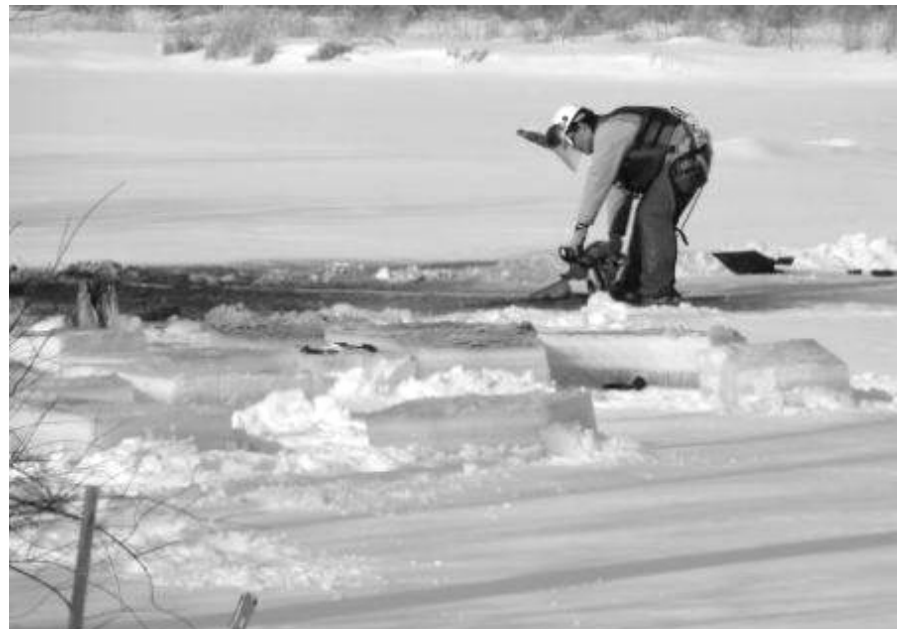
Work crews removed oil from the frozen Kalamazoo River. Additional cleanup of last summer's Enbridge oil spill will pick up this spring and continue into the summer months.
