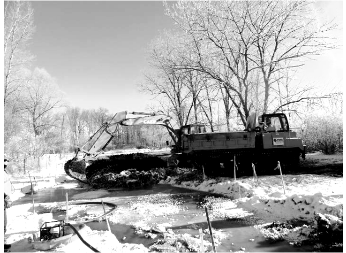
Cold weather solidified the oily sludge and made removal easier. Water was drained from the frozen mixture before disposal and in some cases, recovered oil was recycled.
