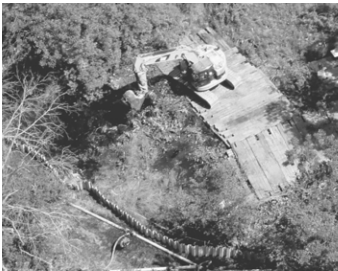
Temporary roads and platforms are constructed so heavy equipment can be brought in to excavate oil-contaminated soil along the Kalamazoo River.
