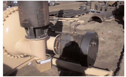
Auxiliary Burner Unit. Photo Courtesy of EnCana.
