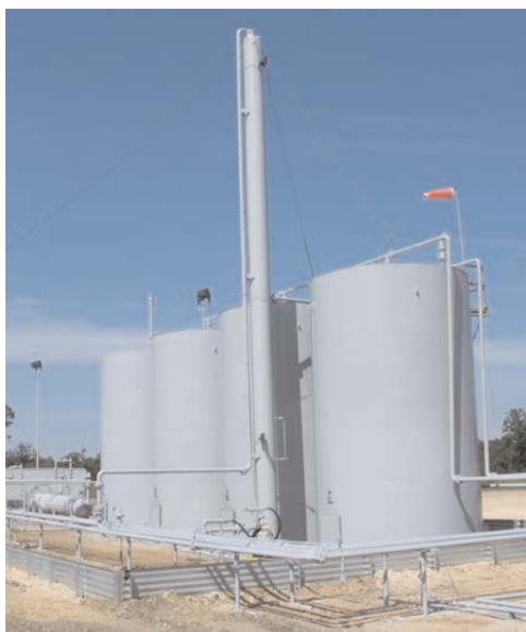
Vapor Recovery Tower. Photo Courtesy of Anadarko.
