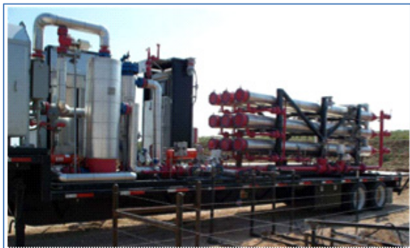
Exhibit 3: CO 2 separation unit (portable membrane system) at a gas well site.
