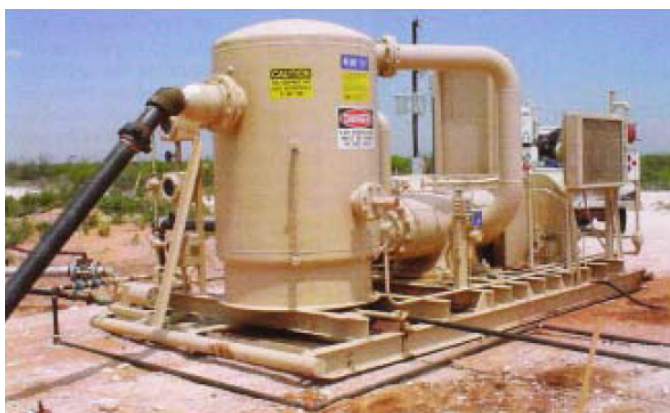
Exhibit 3: Flow lines from multiple wells linked to a single compressor package. Distance is a key consideration before implementing this method of recovery (Source: Hy-Bon Engineering).
