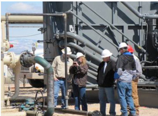
Exhibit 1: Workshop site visit attendees inspecting a leak with the GasFindIR camera at Pleasant Valley station.
