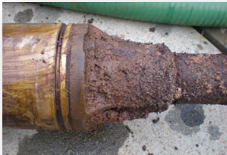
Figure 2. Example of Observed Corrosion on an STP
