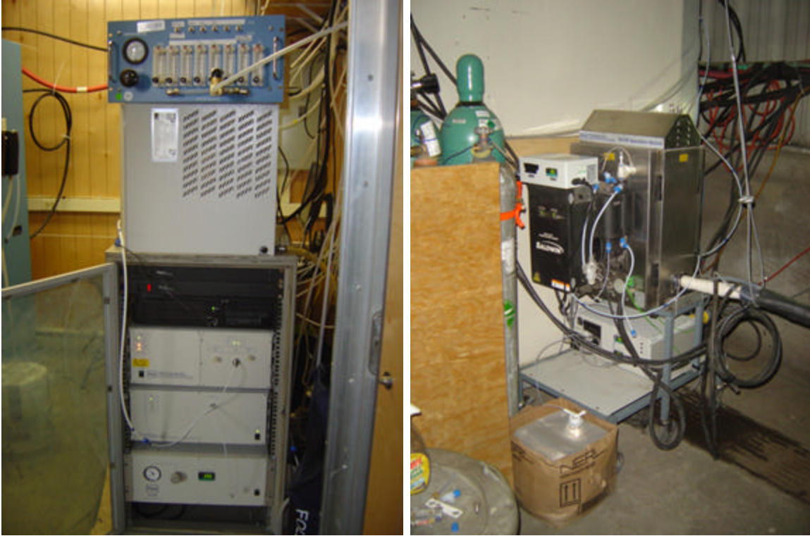
Figure 3-16: GE/PSA CMM Analyzer Located in the CEM Shelter. Its Thermal Converter is Located Outside of the Shelter
