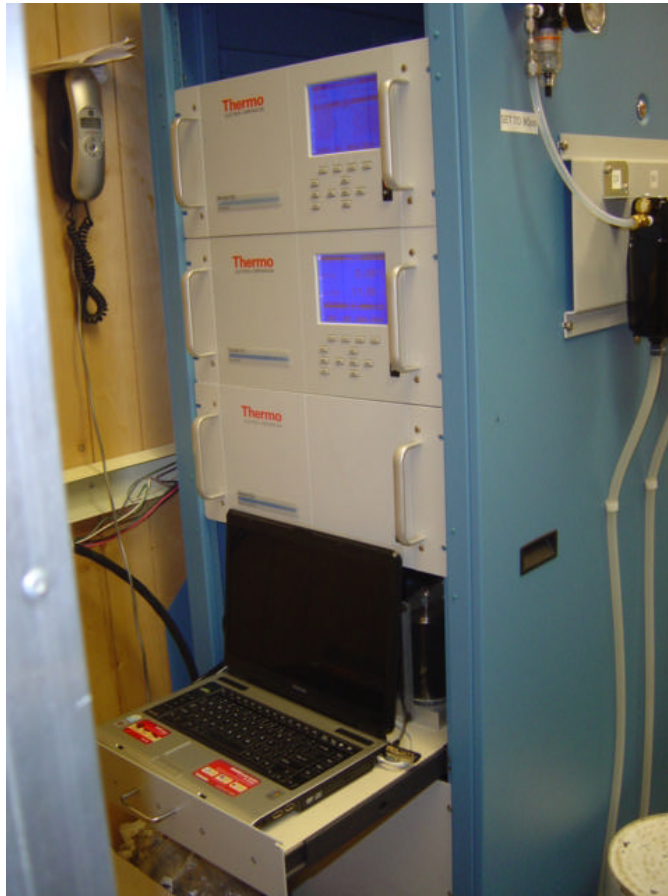
Figure 4-27: Thermo Electron Mercury Freedom System™ at Armstrong
