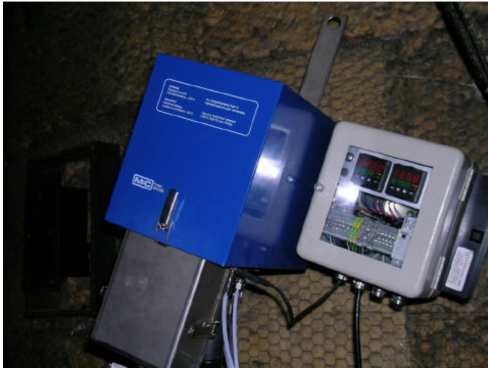
Figure 4-31: Ohio Lumex Probe/Filter/Converter Unit
