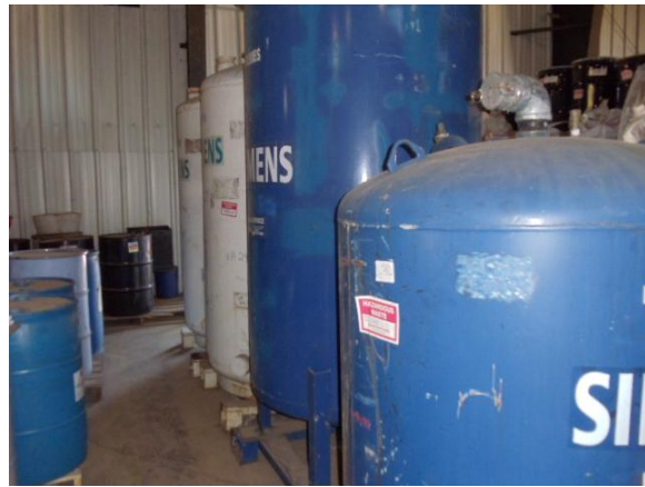
Photo #23: Portable tanks holding hazardous waste spent carbon and clusters in the IS container storage area.
