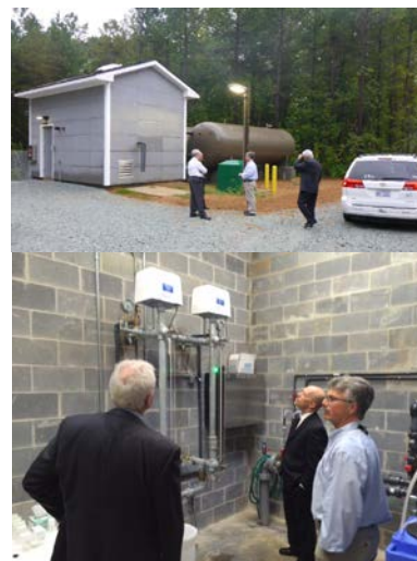
Durham County Public Works Director gave state and federal representatives as well as local press a tour of the new water system location and building
