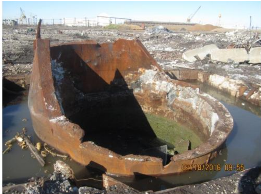
SGS-52 Emergency Relading Pit & Track Scale
