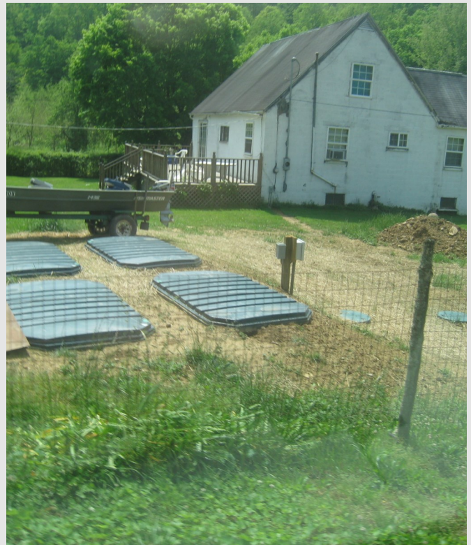
A CWSRF-funded decentralized wastewater treatment system in Lincoln County, West Virginia.
