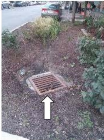
Photo 14-1. An infiltration basin may be poorly sited or poorly designed to the extent that it is unable to retain and infiltrate stormwater. In the photo above, the outlet is too low as evidenced by the scour path from the curb cut to the grate. This could indicate that sediment is being carried into the drain and that little water is being retained and absorbed. Possible solution: consider adding diffuser along scour path and/or raising the level of the grate. (Credit: EPA Region 5)
