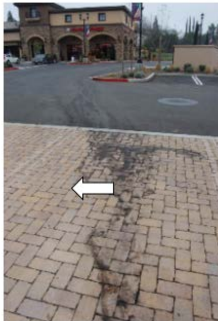
Photo 14-5. Sediment from the impervious parking is entering the permeable pavement area. This photo also indicates improper grading, with the flow accumulating in one area. (Credit: Bill Hunt, NCSU)
