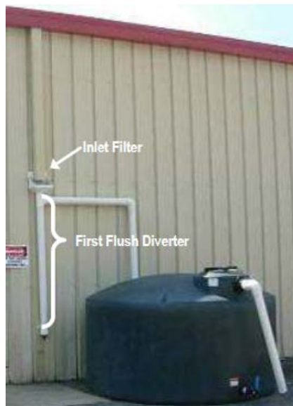
Exhibit 14-10. First Flush Diverter (Credit: NCSU BAE)
