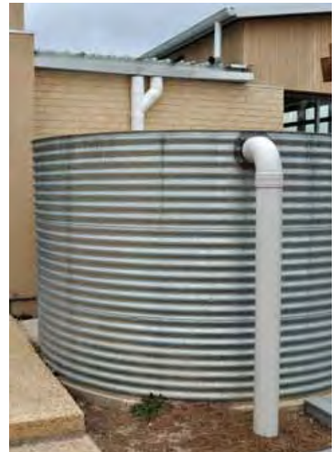
Rainwater collection system
