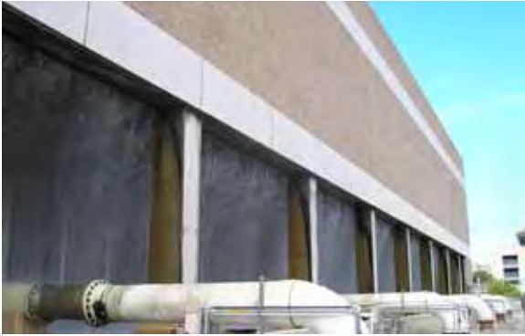
A chilling station making chilled water to cool campus buildings
