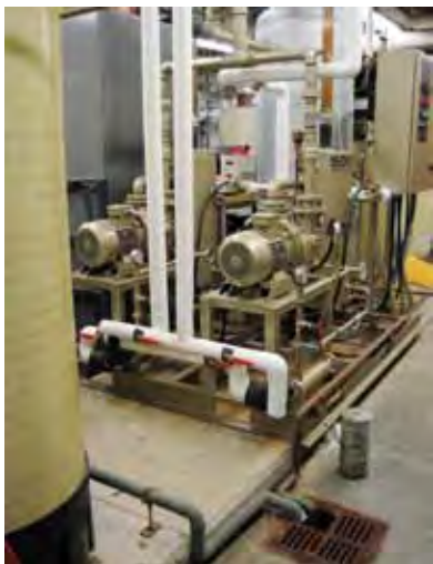
Vacuum pumps at the Kansas City Science and Technology Center
