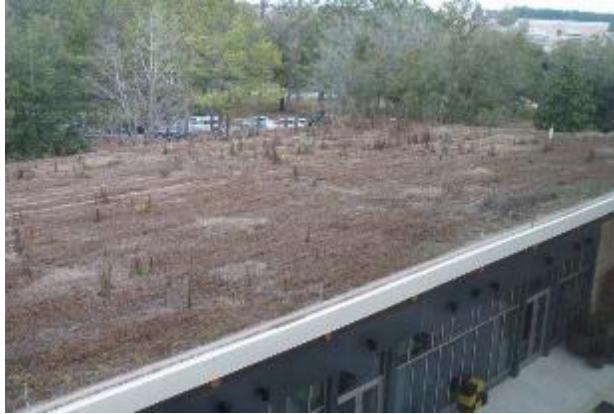
Roof in Florida with poorly maintained plants (Credit: Kevin Songer)
