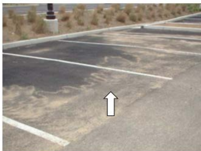
Photo 14-7. Sediment on permeable pavement clogs void spaces thus slowing infiltration. Important to protect permeable pavement from construction stormwater run-off. (Credit: Bill Hunt, NCSU)
