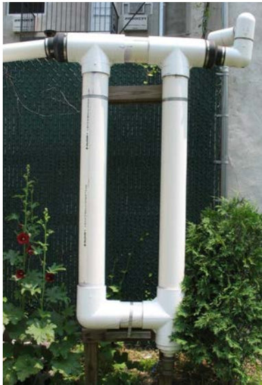
Exhibit 14-11. Roof Washer (Credit: NCSU BAE)
