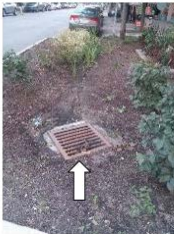
Photo 14-1. An infiltration basin may be poorly sited or poorly designed to the extent that it is unable to retain and infiltrate stormwater. In the photo above, the outlet is too low as evidenced by the scour path from the curb cut to the grate. This could indicate that sediment is being carried into the drain and that little water is being retained and absorbed. Possible solution: consider adding diffuser along scour path and/or raising the level of the grate. (Credit: EPA Region 5)
