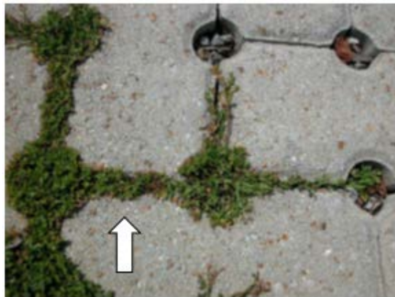
Photo 14-9. Weeds and moss between pavers may indicate a sediment problem. Herbicides should not be used on permeable pavement systems. (Credit: Bill Hunt, NCSU)
